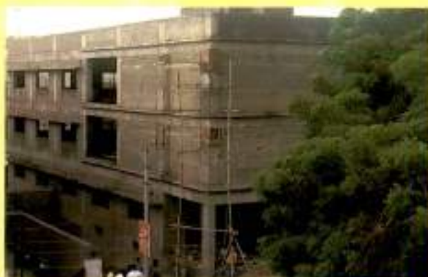
Commercial Building (under construction) on Plot No.299 in Ward 12-B at Gandhidhan.
